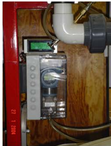
Fig. 6: Elbow-type flowmeter under testing
