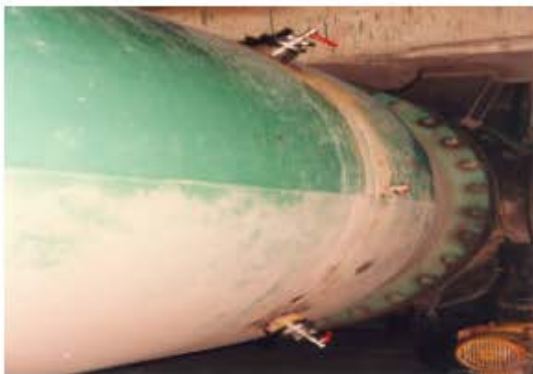
Fig 2: Mounting arrangement of averaging probes in pipeline
