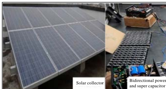
Fig. 12: Equipment of solar panel and super capacitor
