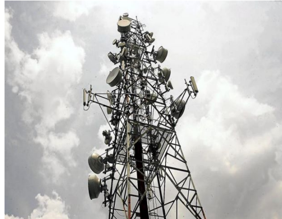
Fig. 1: Example of base transceiver station tower
