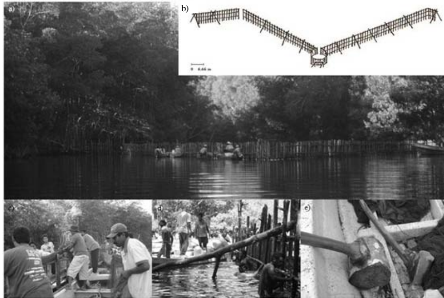
Fig. 2: Construction of the tapo (shrimp corral or barrier) in Lagoon Panzacola: a) A group of fishermen around the tapo still under construction wait for the start of the second and final cooperative workday; b) Figure representing the finished tapo; c) Setting up the tarred mesh on the frame made of wooden parts of varying dimensions; d) Divers place sacks of sand to press the tarred net against the frame; e) Mallet made from red mangrove ( Rhizophora mangle ), one of the handmade manual tools used in making gear; Photos c and d denote a type of cooperative division of labour
