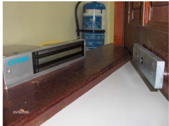
Fig. 2: Door with electromagnetic lock
