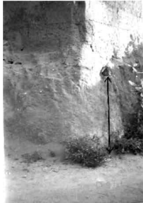
Fig. 2: Foundation of a mudhouse exposed by 1.2 m (shown with arrow) by sheet erosion and street floods over duricrust concretions within the built-up areas (site A in Fig. 1)
