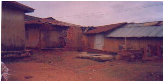
Fig. 13: Structurally and qualitatively deficient buildings, jumbled together in Isale Osun area (Researcher’s field work, 2018)
