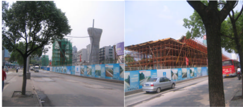
Fig. 2: Cross-road (interchange) construction at the junction of Zhuo Dao Quan and Luo Yu roads in Wuchang
