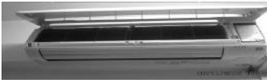
Fig. 5: Measure cooling coil temperature
