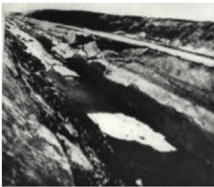
Fig. 1: Example of disorders in the construction of «Samour-Apchéron» concrete channel
