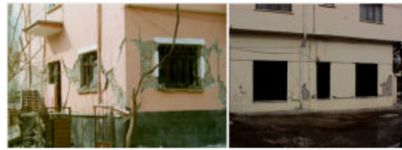
Fig. 10: X Cracks in a masonry structure
