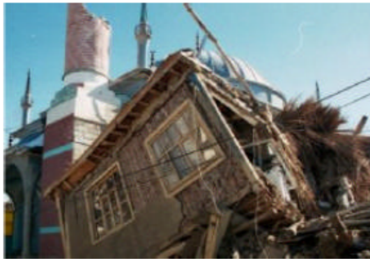
Fig. 9: Highly damaged non-engineered structure
