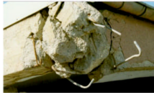
Fig. 5: Insufficient material and detail in a joint
