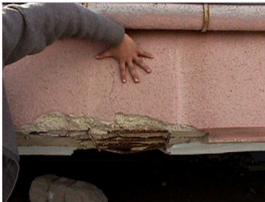
Fig. 4b: Insufficient material and detail in a column
