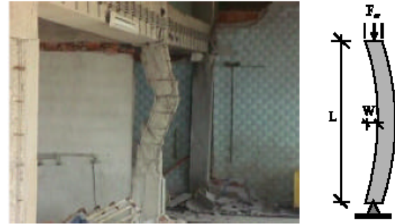
Fig. 7: Buckling column damage in industrial facility of Cay
