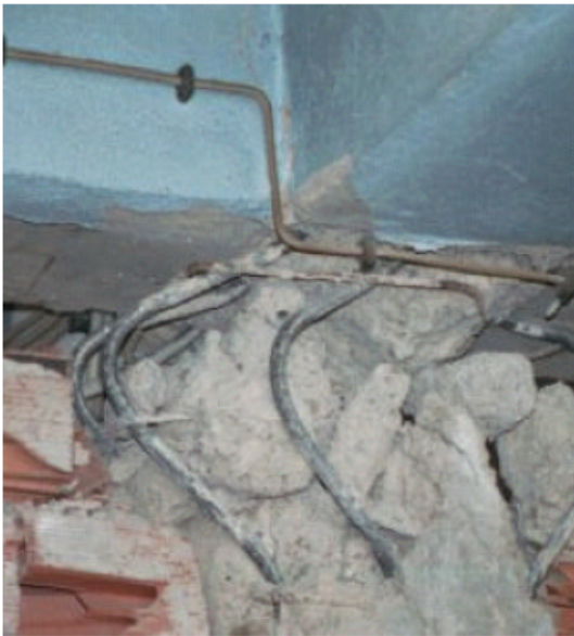
Fig. 6: Insufficient material and detail in a column
