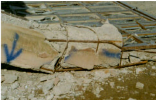
Fig. 4a: Insufficient material and detail in a beam
