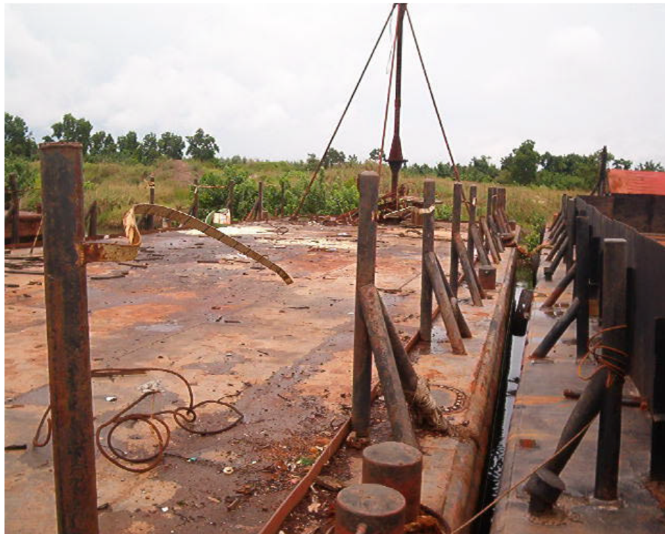
Plate 1: Typical deck plate condition for a work barge in service
