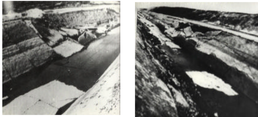
Fig. 1: Example of disorders in the construction of « Samour-Apchéron » concrete channel
