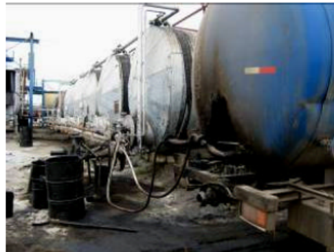
Fig. 7: A view of pipes connections used to supply heat to flowing bitumen (Courtesy: Julius Berger Nig. Ltd.)
