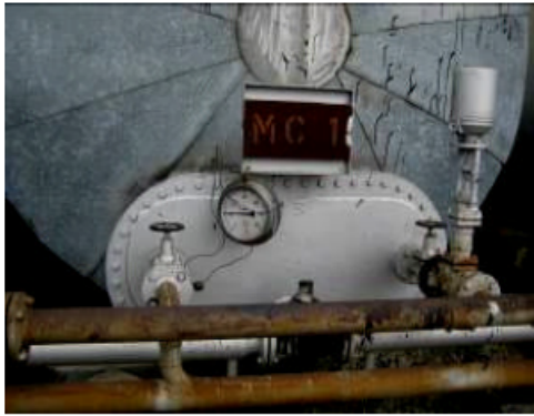
Fig. 8: Tank designated for the production and storage of MC1
