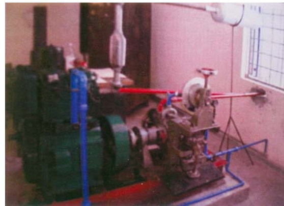
Fig. 3: Actual image of converted diesel engine
