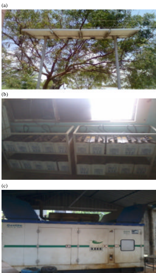
Fig. 10: The photograph of the experimental setup for: a) Solar panel; b) Battery bank; c) Generator
