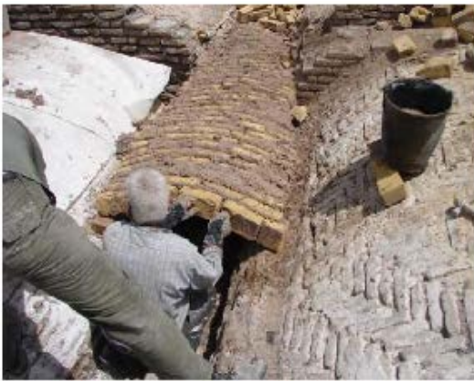
Fig. 18: Implementation of queuing between two cadence arches in Saraye Dokhan of Zanjan
