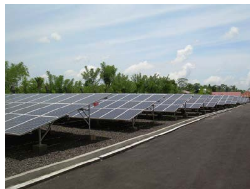
Fig. 1: The PV system
