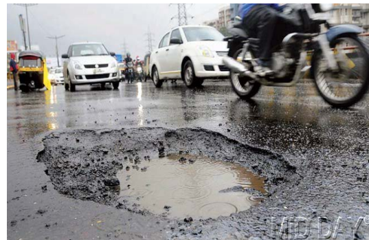
Fig. 1: Roads condition with potholes
