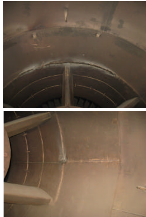
Fig. 1: A view from inside of the diffuser examined and location of the temperature sensor and repaired welds
