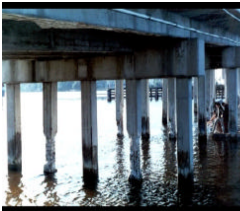
Fig. 1: Structural damage (chabahar harbor)
