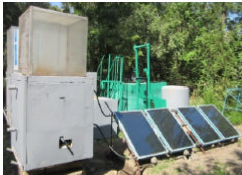
Fig. 3: General view of the solar
