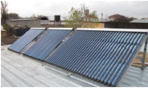
Fig. 2: Tubular solar collector
