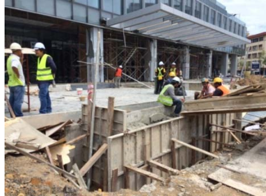
Fig. 5: Inadequate safety supervision
