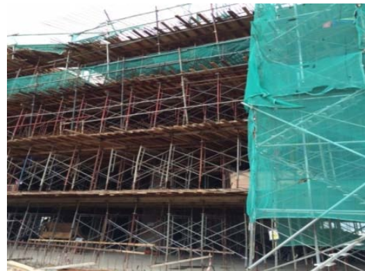
Fig. 1: Inadequate safety measures
