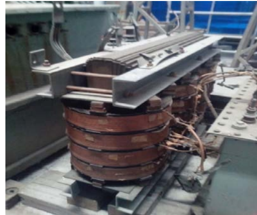
Fig. 4: Site power transformer as a case study
