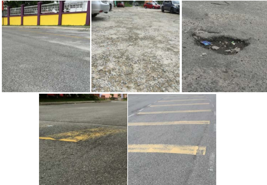
Fig. 2: Road surface conditions from left, smooth surface, uneven surface, pothole, speed bump and hazard lines
