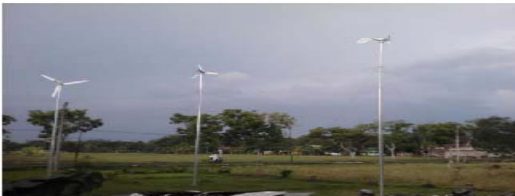
Fig. 8: The installed 1.2 kW wind power system
