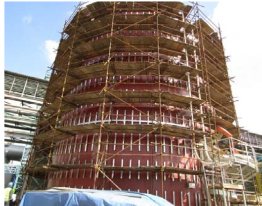
Fig. 1: Steel tank for the storage of limestone suspension
