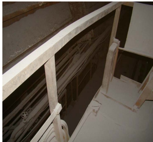
Fig. 9: The absence of the guard rail middle element
