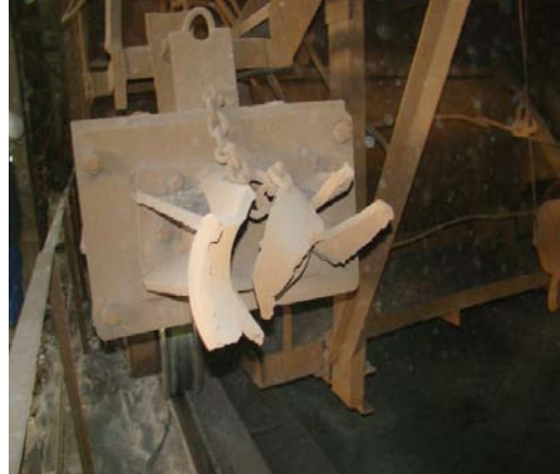
Fig. 7: Bridge crane stop destruction
