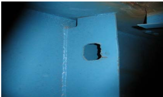
Fig. 11: Non-standard holes in the transverse stiffeners
