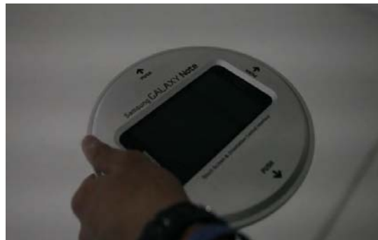
Fig. 19: Installed 'Galaxy Note' controller
