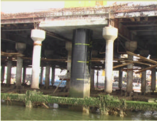
Fig. 2: The process of constructing 46 inch reinforcing pile to improve seismic behavior of East Wharf of Imam Khomeini Port
