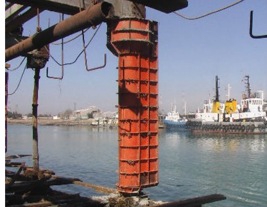
Fig. 3: The process of constructing concrete jacket to improve seismic behavior of East Wharf of Imam Khomeini Port
