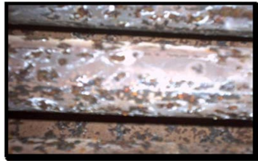
Fig. 6: Pitting corrosion inside boiler (Roberge, 2000)
