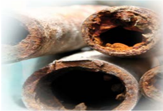
Fig. 4: Scale inside boiler tubes (Roberge, 2000)
