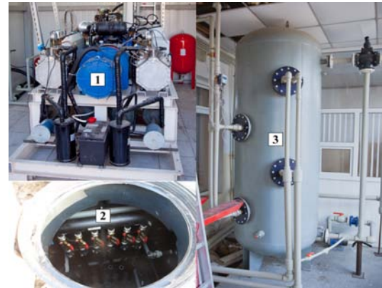
Fig. 11: Experimental polygeneration plant
