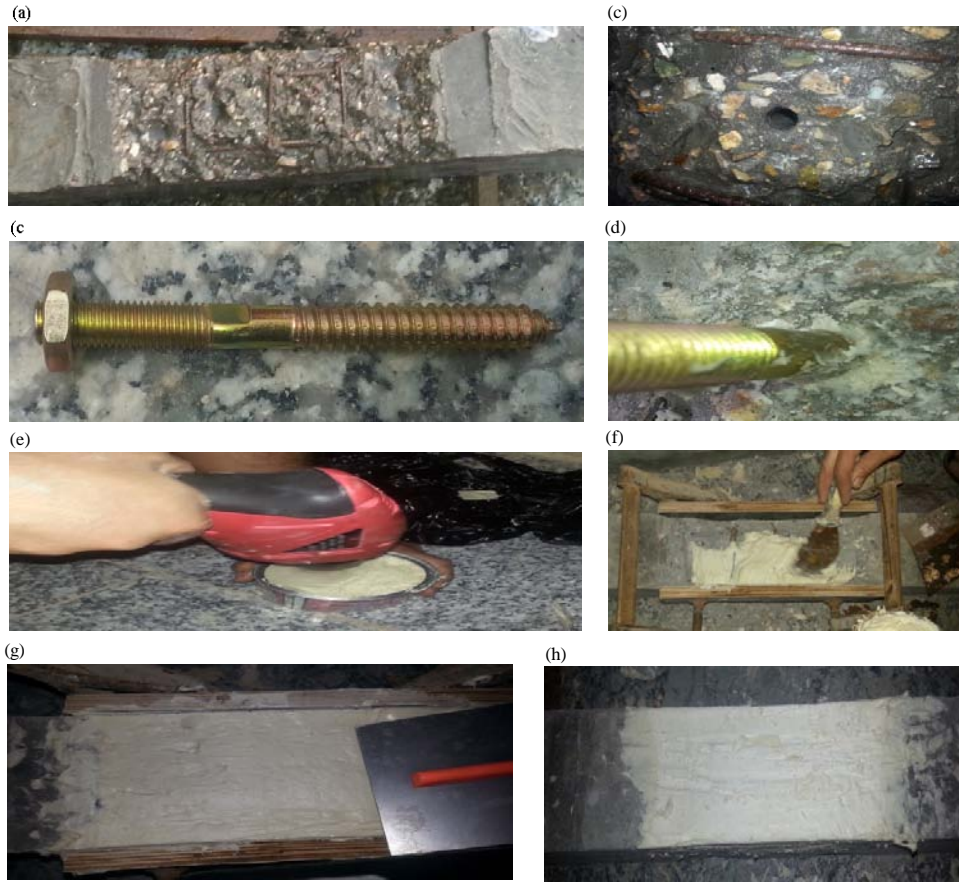
Fig. 4: Repairing with polyester glue line: a) Clean the damaged zone; b) Hole of shear connector; c) Shear connector; d) Fixed shear connector; e) Mixing polyester glue line; f) Pervading polyester glue line; g) Adjustment polyester glue line and h) Repaired damaged zone
