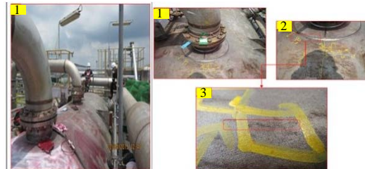
Fig. 5: General view top shell from east plant side. 1-3 typical finding as above
