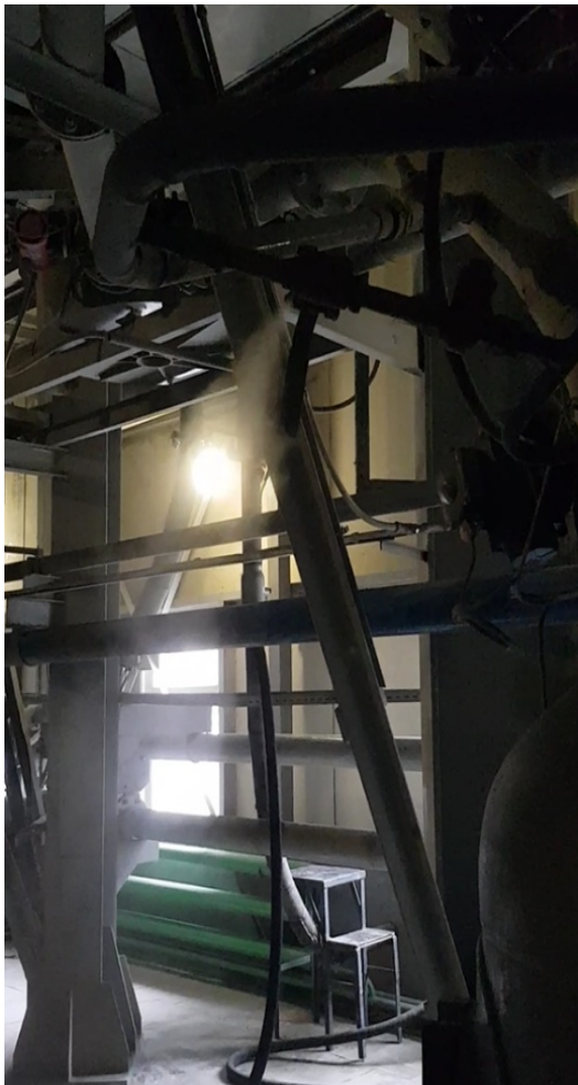
Fig. 2: Crack in a metal pipe
