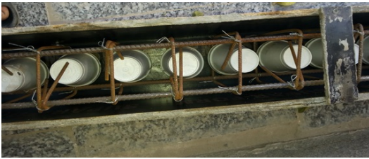
Fig. 2: Conic voids inside steel cage
