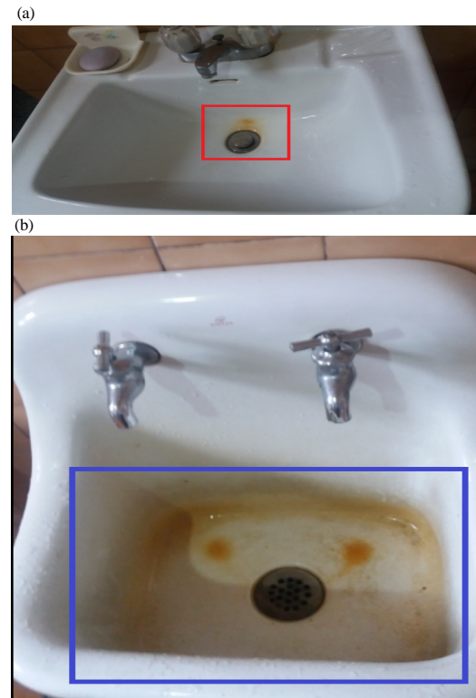
Fig. 1: Example of water in undrinkable heavy metals: a) heavy metals at red position and b) Heavy metals at blue position
