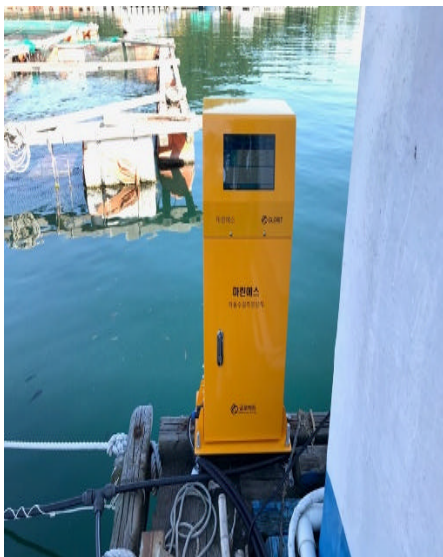
Fig. 3: Marine-S smart water quality measuring sense
