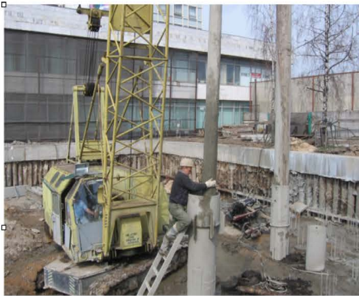
Fig. 4: Structure of bored piles in saturated sands on the left-installation the bailer for excavating from the casing of biogenic soils over the compacted ground plug to the right-its displacement by a second pipe with closed end
