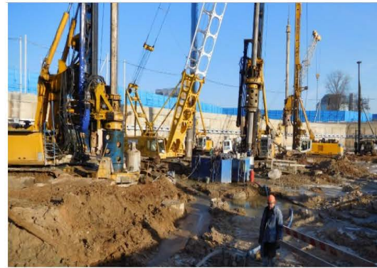
Fig. 5: Drilling of wells by drilling rigs of the firms "Bauer" and "Cassagrande" under the protection of casing pipes with scooping out of the ground by bailers and refilling of water into the casing
