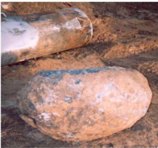
Fig. 12: The cases-punch with butt plugged end and excavated rammed pedestal under the pile toe
