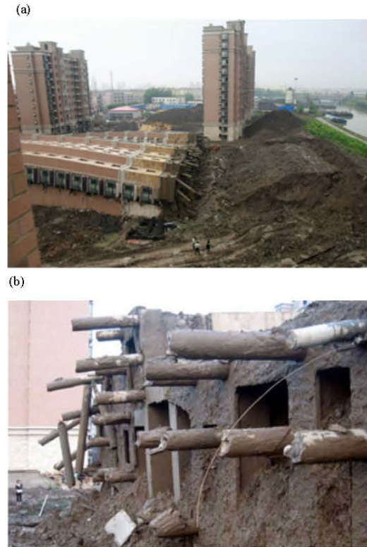
Fig. 3a, b: Collapsed in Shanghai, a 13 storey residential building (Anonymous, 2009) in the failure of prefabricated hollow reinforced concrete piles, weakly reinforced by tensile rods of small diameters
