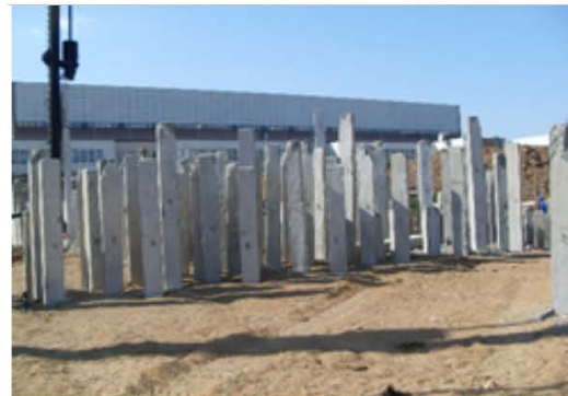
Fig. 2: Not be driven to design marks of piles
