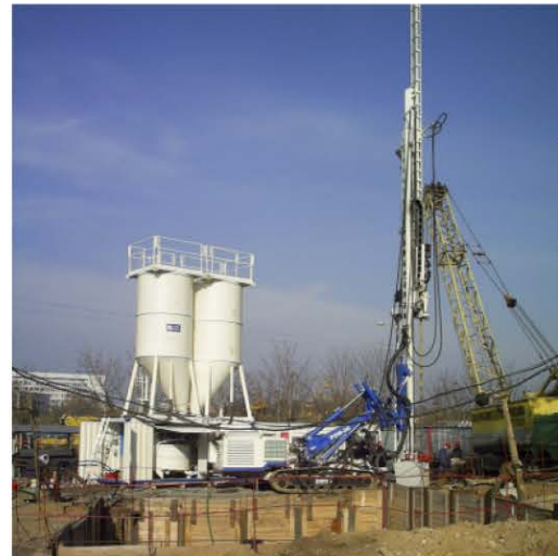
Fig. 18: The equipment of Italian company soilmec for inject technology
