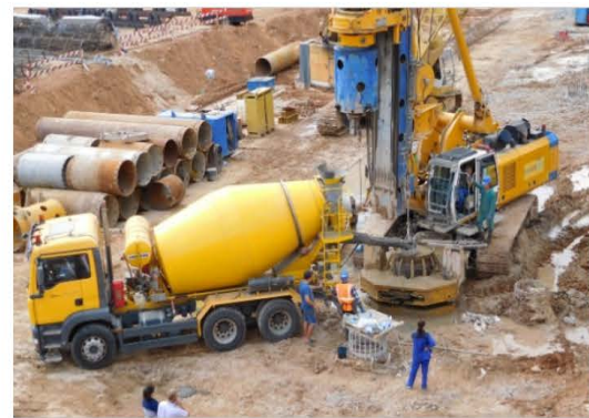
Fig. 6: Concreting of piles in a casing filled with water by the method of VPT when pouring concrete from a mixer through the socket of a concrete pipe
