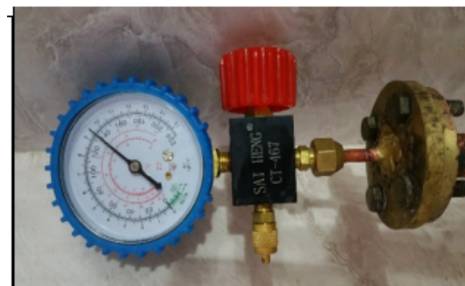
Fig. 4: Gauge on heat pipe condenser
