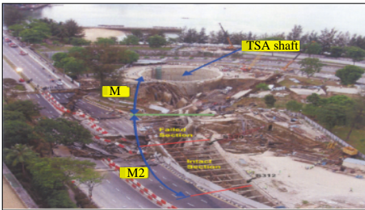
Fig. 3: The collapse of Nicoll Highway, Singapore on 20th April 2004. (Proc. 16th South East Asian Geotechnical Conference)
