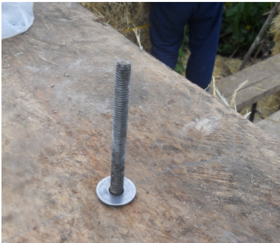
Fig. 12: Detail of the joint between the wooden planks and the bales the screw is missing
