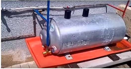
Fig. 2: Geyser with temperature sensors and control
