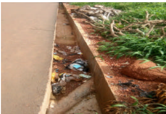
Fig. 11: Underlying pipe cutting across the drainage system in University-Road
