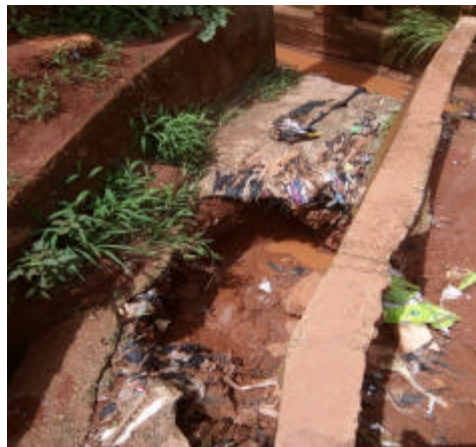
Fig. 9: Sections of failed drainage system in University Market-Road
