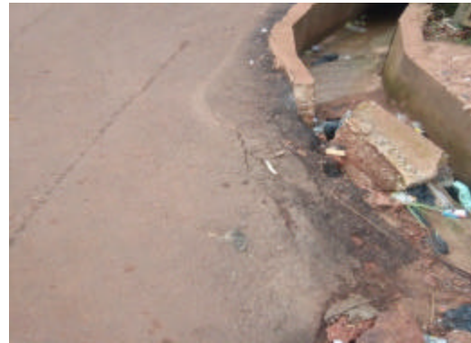
Fig. 8: Section of poorly constructed drainage system in Odenigwe-Road
