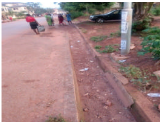
Fig. 7: Section of poorly constructed drainage system in Aku-Road
