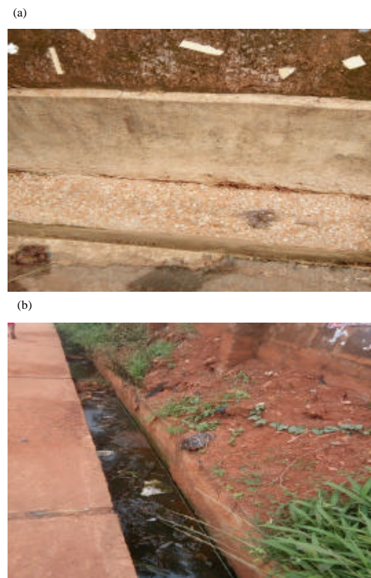
Fig. 24: a) Stone pitching method at University Market-Road and b) Un-stone pitched soil mass in Odenigbo Road
