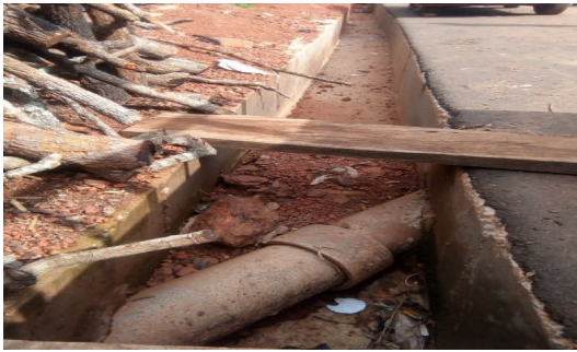
Fig. 10: Underlying pipe cutting across the drainage system in Odenigwe-Road and University-Road
