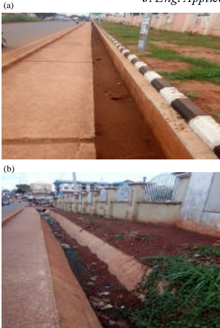
Fig. 25: a) Cementing method with kerb in Odenigbo Road and b) Un-cemented soil mass at Enugu Road
