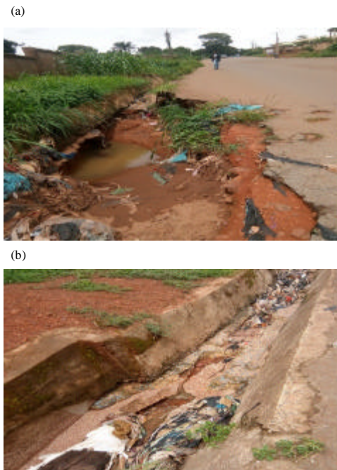
Fig. 22: a, b) Roads with temporary waste site, very poor waste managements and poor drainage condition, e.g., University market-Road
