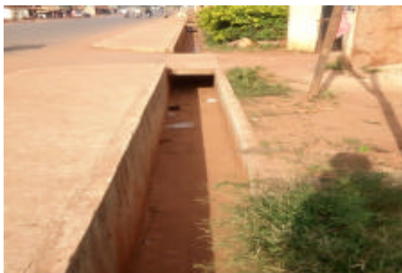
Fig. 17: a) Roads with good waste management, good drainage condition and without temporary waste site in Enugu Road and b) Roads with good waste management, good drainage condition and without temporary waste site in Orba Road
