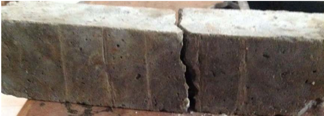
Fig. 3: Beam showing crack after failure due to bending
