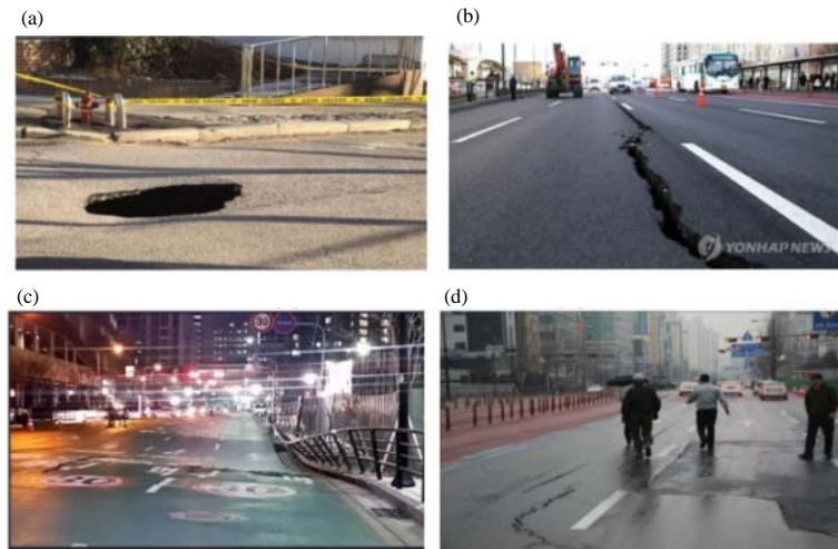
Fig. 3: Ground sinking occurrence site in the OO area in South Korea: a) First ground sinking; b) First road crack; c) Second road crack and settlement and d) Third road crack
