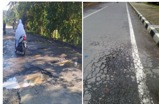
Fig. 1: Expansive soil conditions on the Takalar-Jeneponto highway
