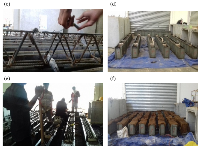
Fig. 4(a-f): The process of specimen installation, (a) Bar welding assembly, (b) Truss system reinforcement, (c) Strain gauge, (d) Formwork, (e) Casting and (f) Curing
