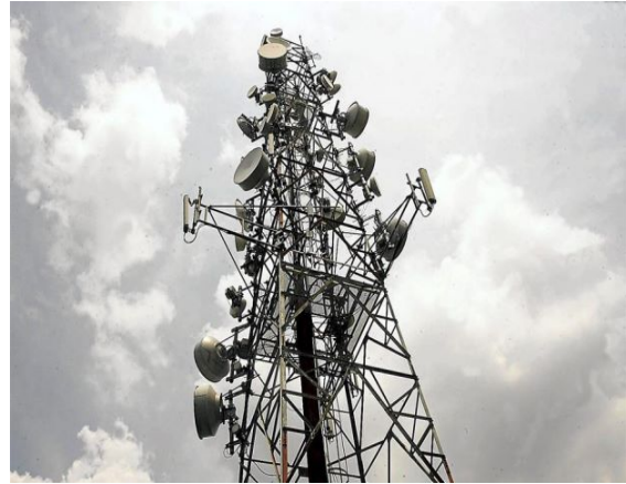
Fig. 1: Example of base transceiver station tower
