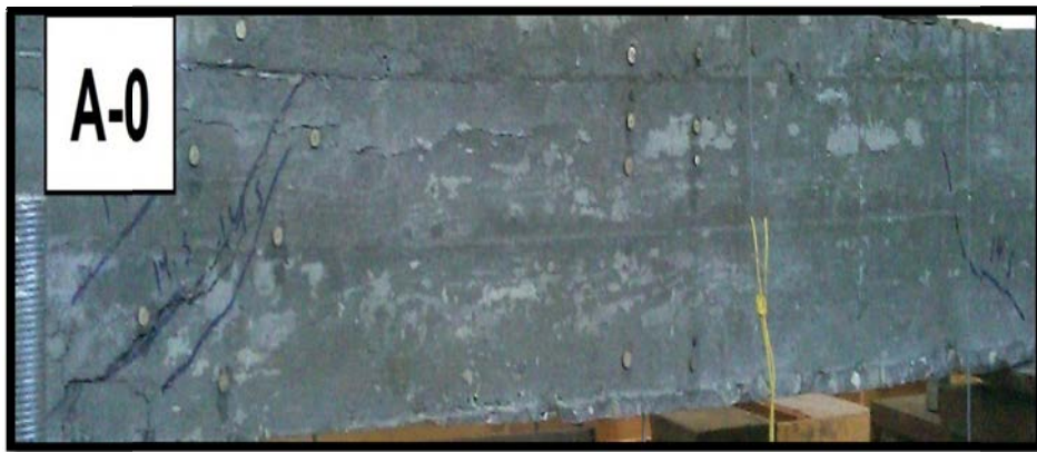
Fig. 7: Crack patterns for specimen (A-0)
