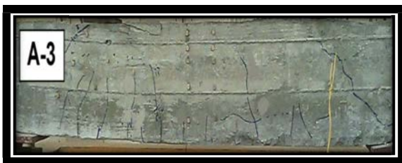
Fig. 16: Crack patterns for specimen (A-3)
